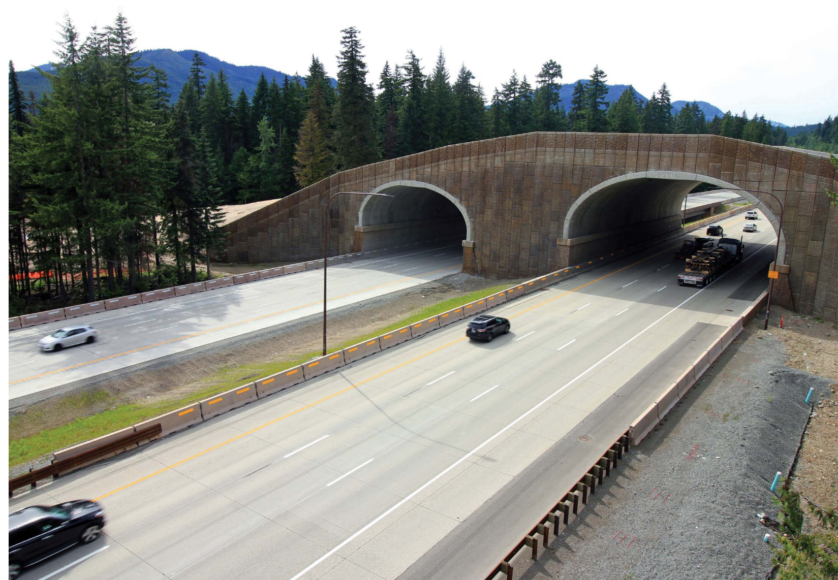
The key to ensuring wildlife use overpasses is directing them with roadside fencing. Photo by Washington State Department of Transportation
